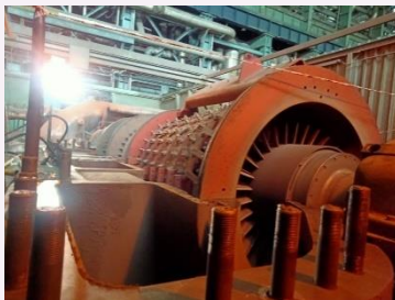
OVERVIEW – Turbo blower station
